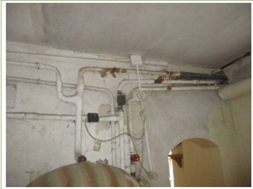
Pipework insulation in the basement kitchen plant room in the main house
