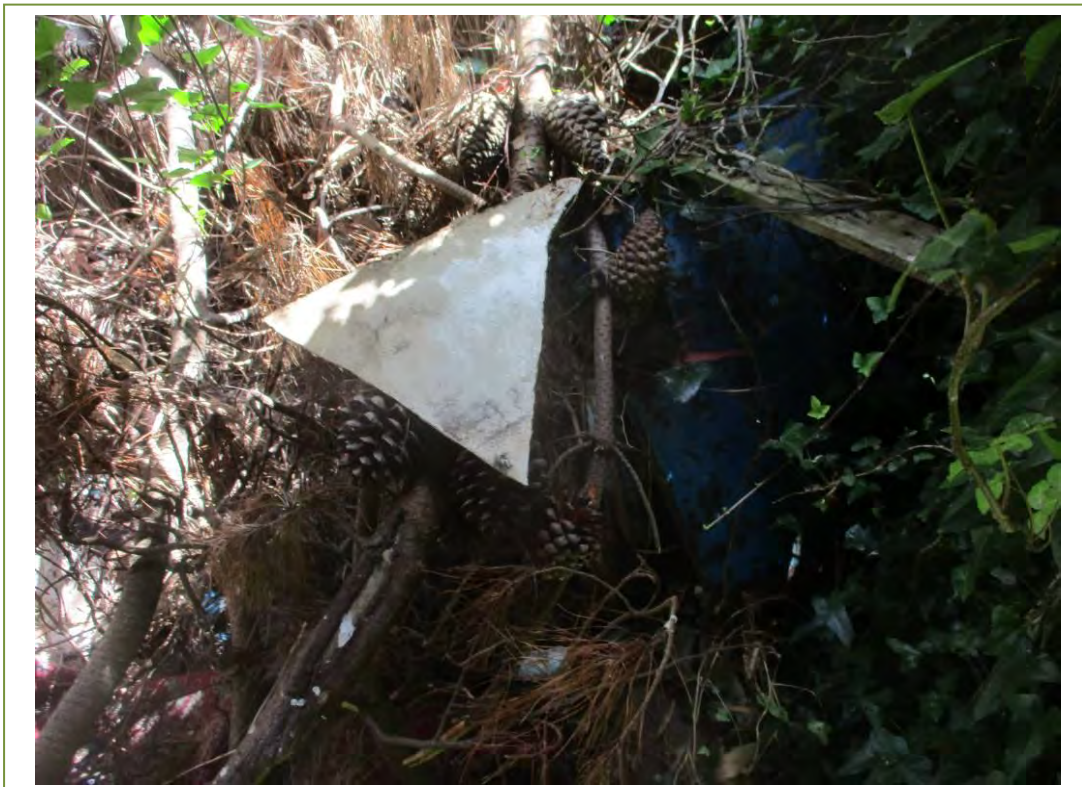
Asbestos cement board debris in the rear derelict building
