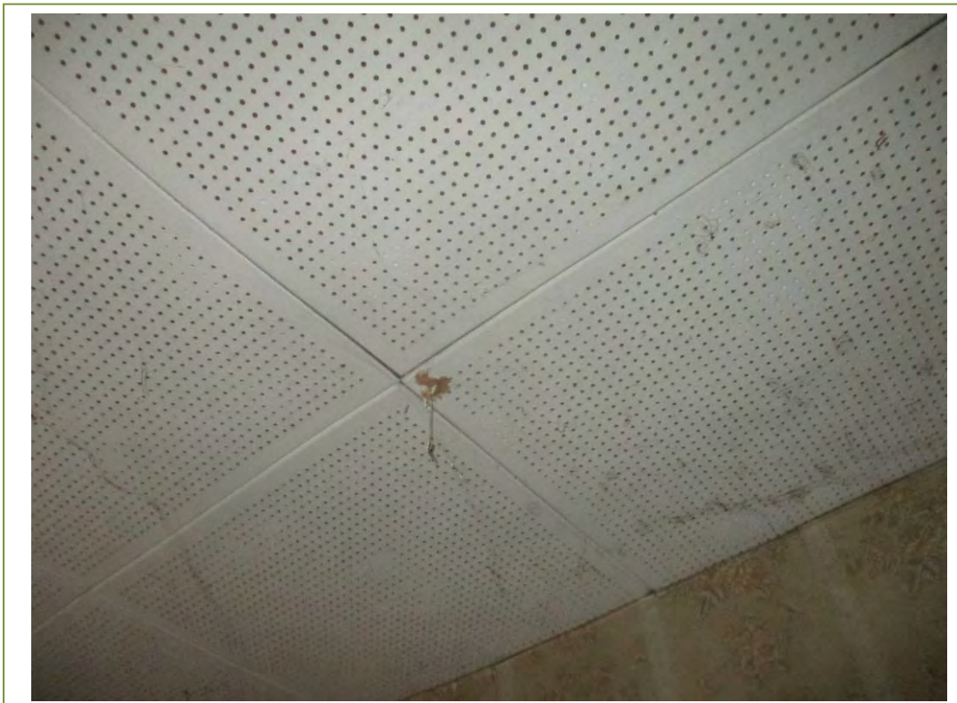
Ceiling tiles in the living room in the gate lodge at the road
