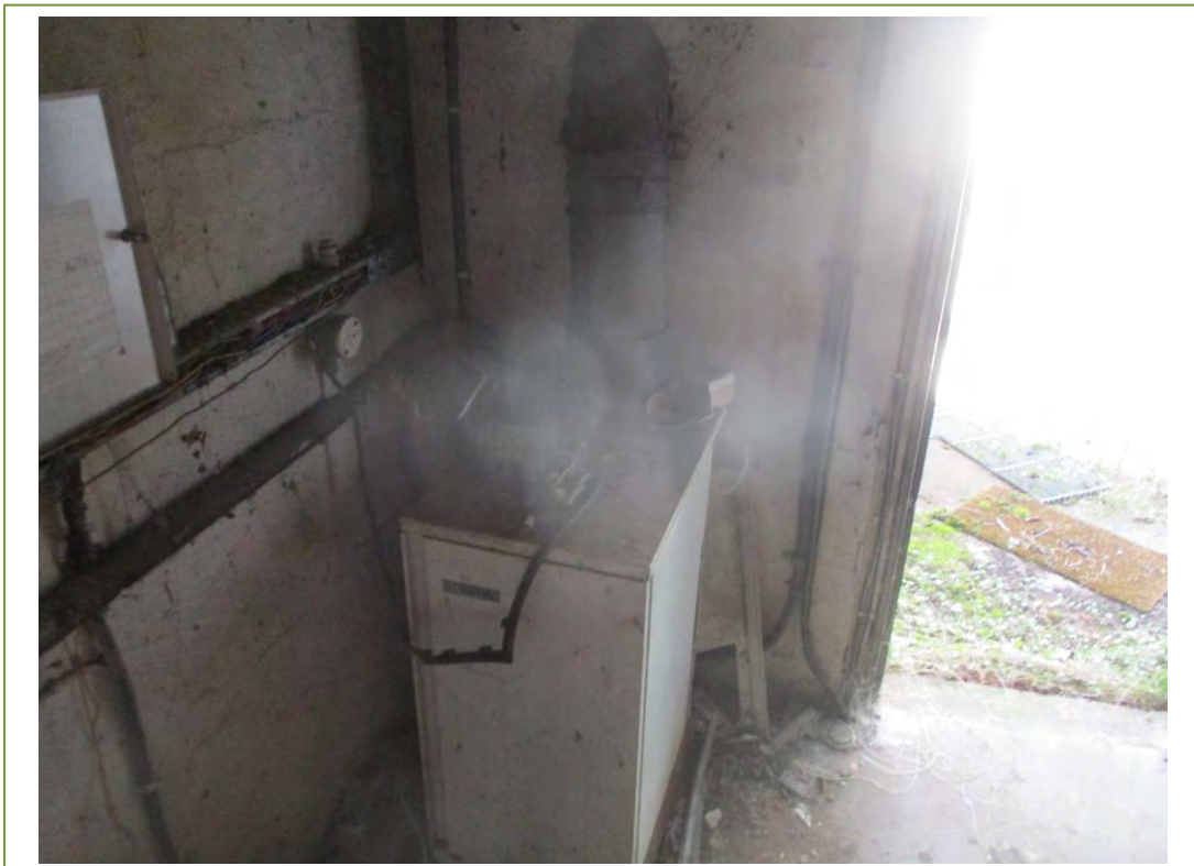
Boiler unit in the external boiler room in the main house
