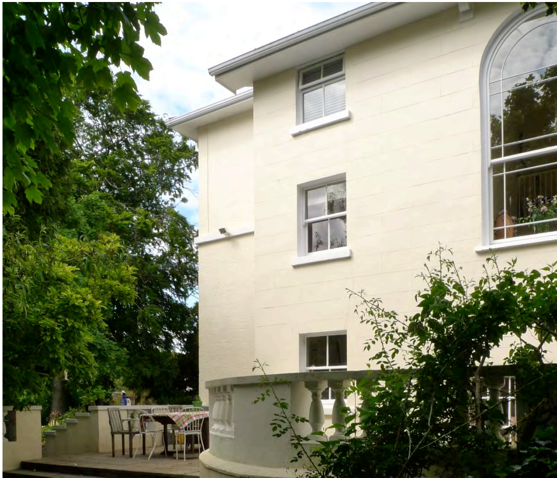
Figure 4.4 Carrickbrennan The south façade, the large window to the stairs would have originally given a composed view of the Dublin Mountains
