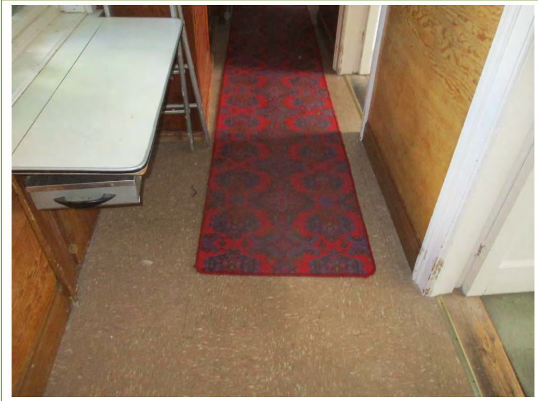
Floor tiles in the corridor on the ground floor in the main house
