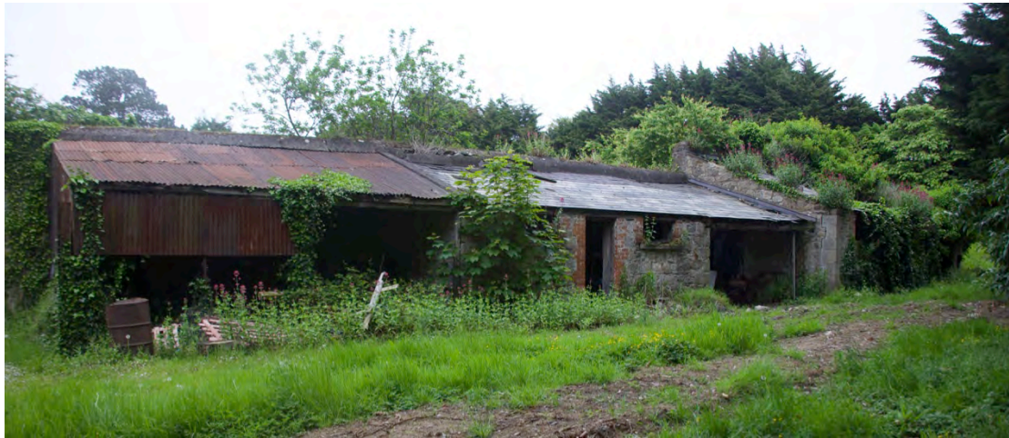
Figure 5.8 The range of bothies outside the southern end of the walled garden
