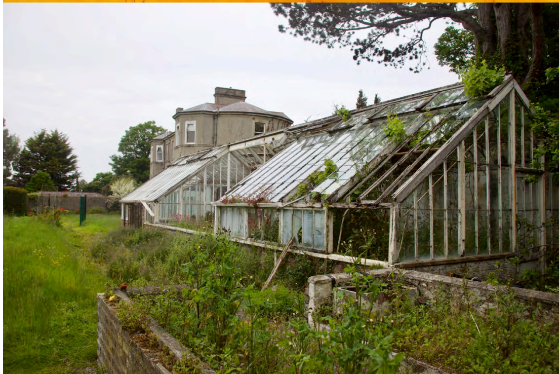
Figure 5.7 The glasshouse, above the design drawing from McCurdy and Mitchell (IAA) and below as built with an extra bay. The first bay was a vinery and the second probably a peach house (there is still a peach tree struggling in this near complete ruined bay)
